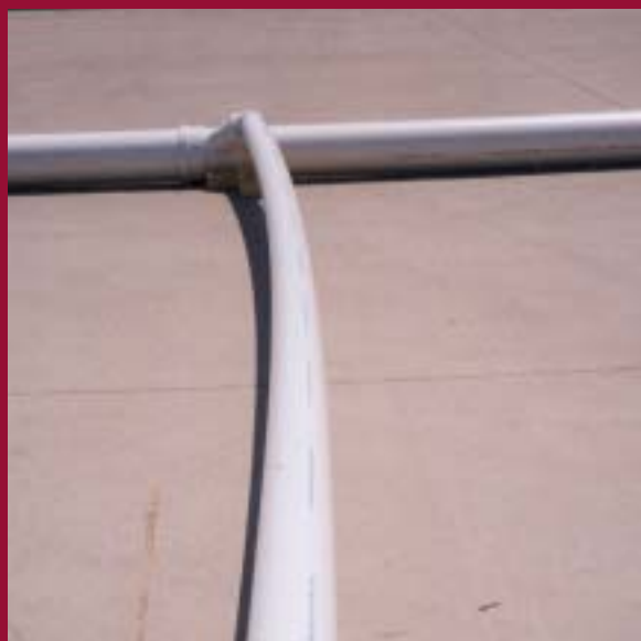
Figure 3 A typical "field adjustment" is photographed here. This "adjustment" produces an extraordinary amount of stress on the fittings.
